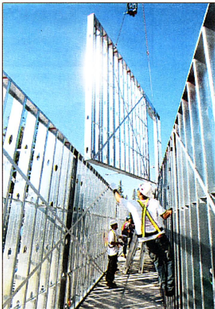
Construction workers move a modular galvanised steel stud wall during the construction of the project.
