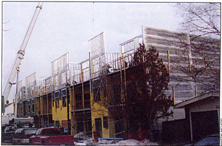
Exterior, corridor, and party wall panel assemblies are built to rigid tolerances on semi-automated panellizing tables using 8", 6" or 3-5/8" LSF.
