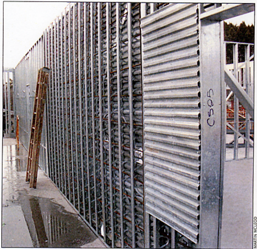
Interior third floor LSF walls being installed with steel framed concrete shear wall in foreground portion.
